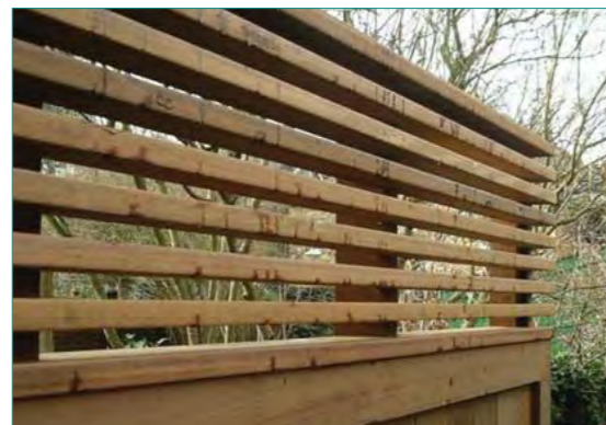
Robust horizontal rail timber screen to edge of riverside square, ht 1.2m
