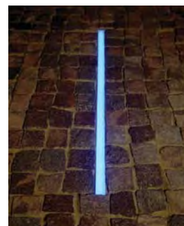
In-ground LED lighting
