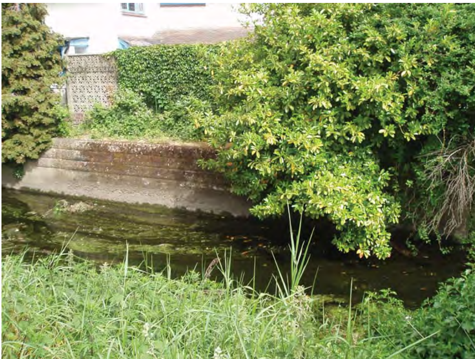
Plate 2: View of River Crane adjacent to the site. Note concrete lined structure.
