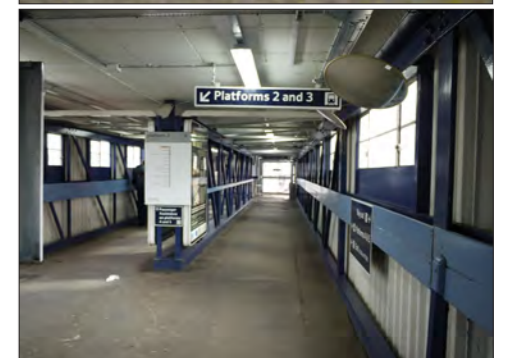
LINK BRIDGE VERY NARROW, POOR INTERNAL ENVIRONMENT AND NEGATIVE EXTERNAL APPEARANCE
