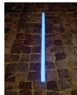
In-ground LED lighting
