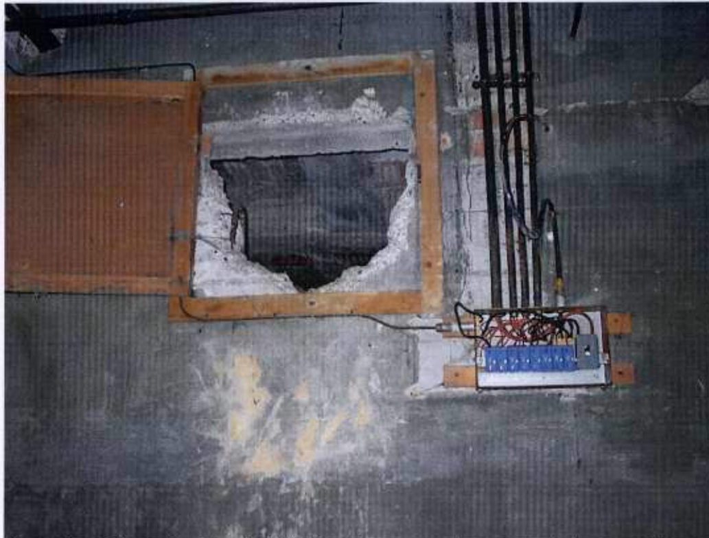
Plate 17 - Changing Block - high level access door to sub-floor void adjacent swimming pool
