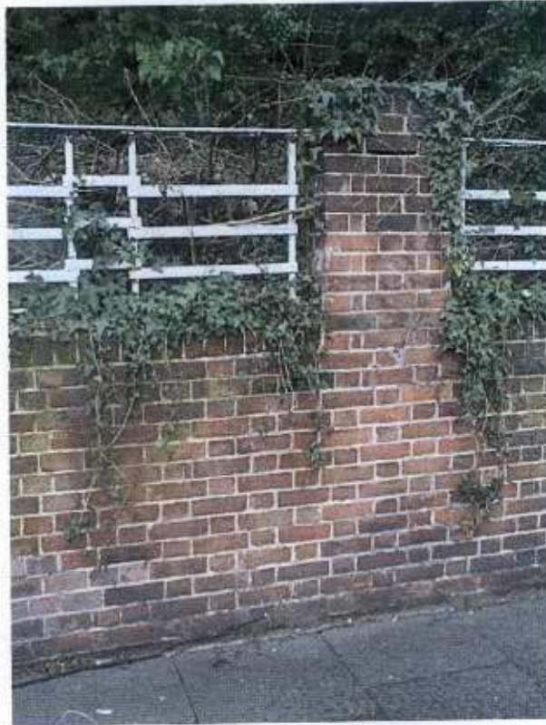
Wall north east of pool building, which will stay as part of proposed garden.
