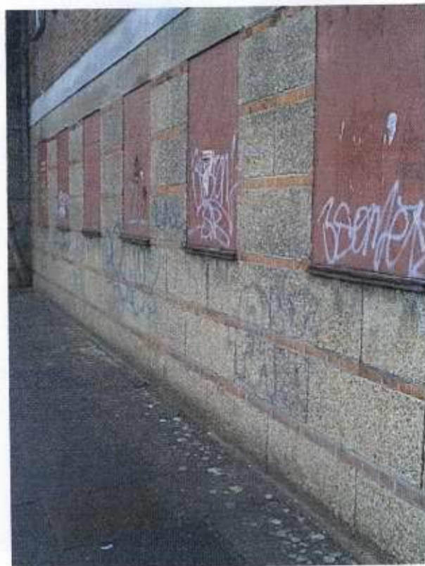
Pool building wall and window, which will be demolished to make way for proposed garden.
