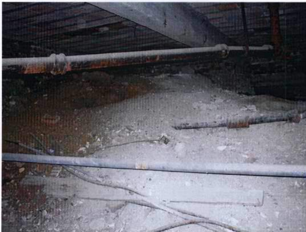
Plate 18 - Swimming Pool - sub-floor void between swimming pool and northeast elevation of changing block
