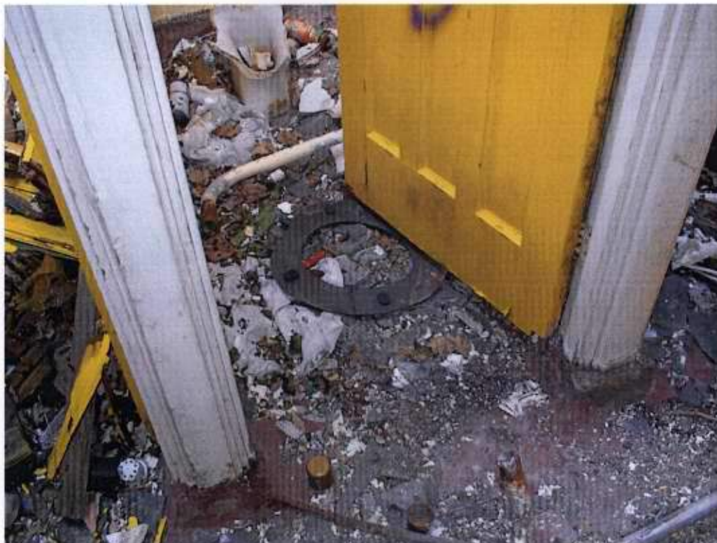
Plate 10 - Changing Block - toilet seat debris to floor of gents WC (West Toilets)
