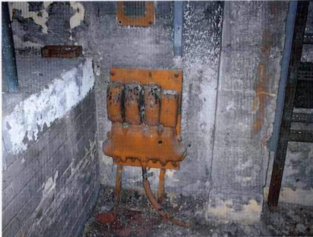
Plate 13 - Changing Block - electrical equipment within northeast plant room on lower level
