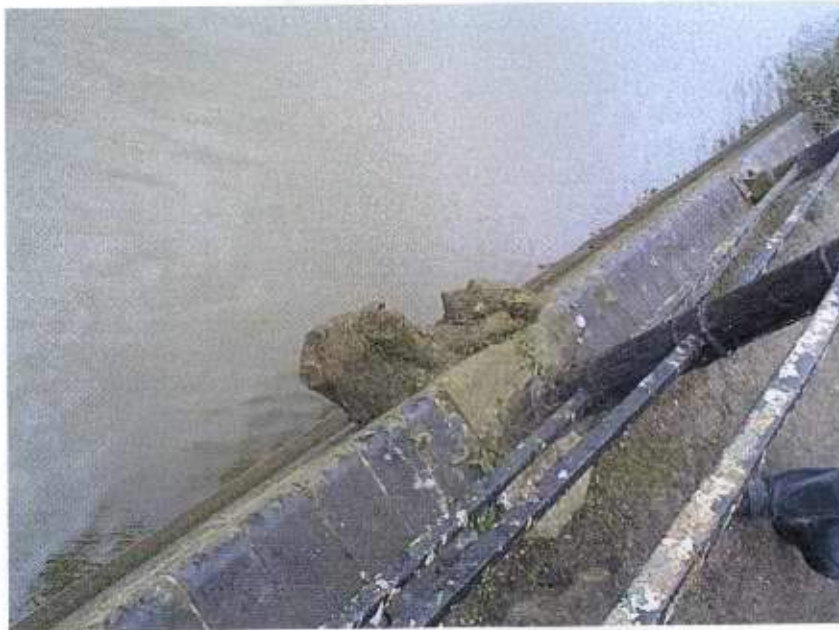
Root through Thames River wall.
