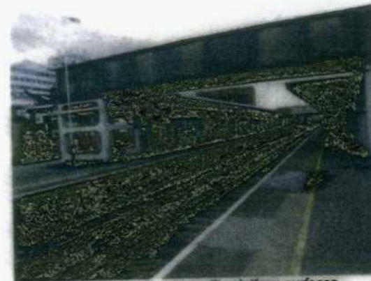
Unightly overbridge & poor quality platform surfaces
