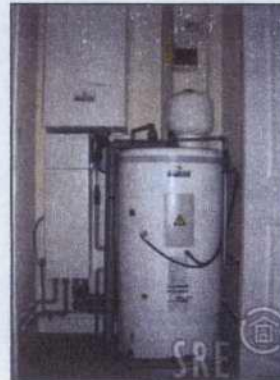
Internal Control Unit and Thermal Store
