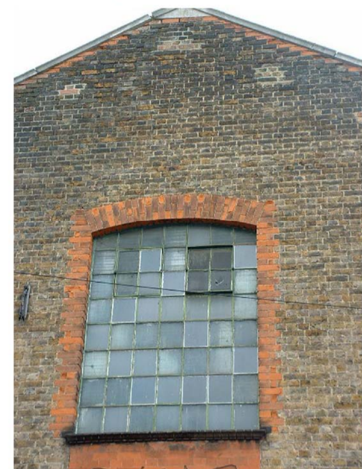
Window reveal quins, arches and decorative window cills to be retained, brickwork to be cleaned
