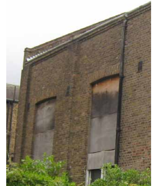
photograph of the existing boarded up windows to the west elevation. Below is a sketch view of the proposed recessed windows with the projecting timber shutters
