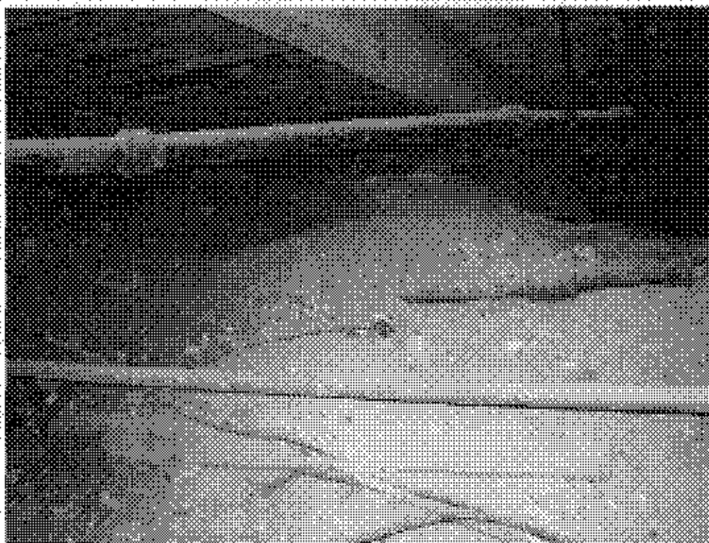
Plate 18 - Swimming Pool - sub-floor void between swimming pool and northeast elevation of changing block
