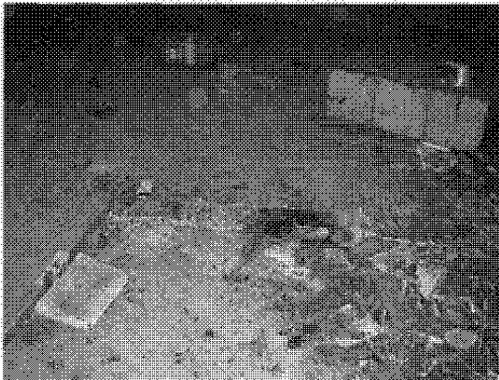
Plate 8 - Changing Blocks - redundant pipe unit in southwest plant room on lower level.
