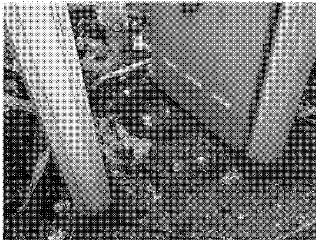
Plate 10 - Changing Block - toilet seat debris to floor of gents WC (West Toilets)
