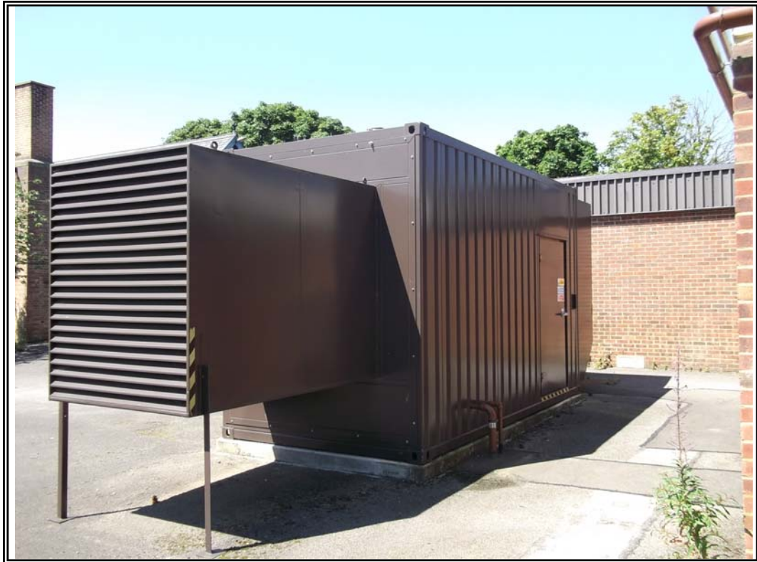
The emergency generator
