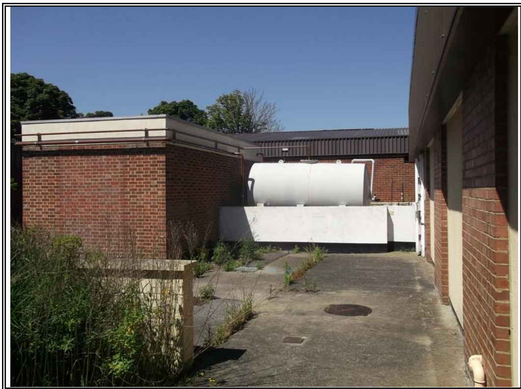
Above ground fuel tank for the emergency generator
