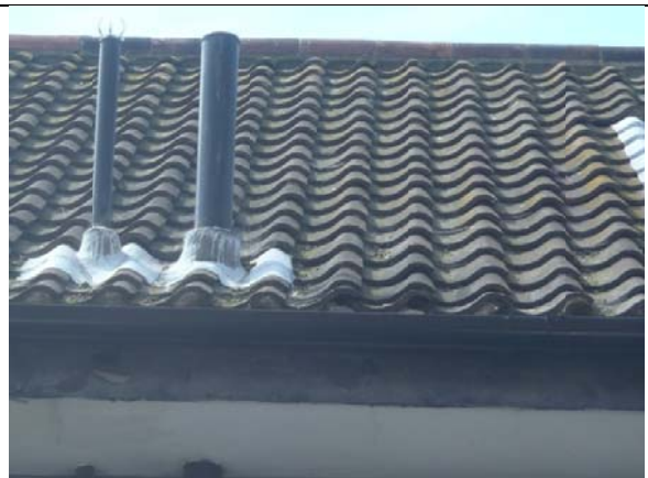
P10. Further occasional gaps under roof tiles above sections of lead flashing on the north eastern side of the roof of Building 3.
