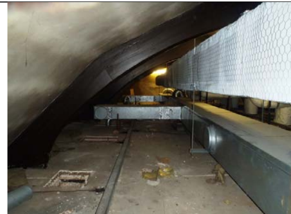
P3. The roof space in Building 2 showing the pipe work and boarding under the roof.
