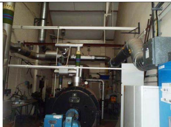
P16. The interior of the boiler room within Building 4.
