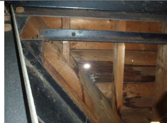
P13. Daylight visible between the sarking boards in the centre of the roof space of Building 3.
