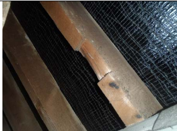
P6. The exposed bitumen and hessian felt at the south eastern end of the void.
