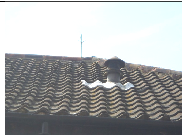
P9. Occasional gaps under roof tiles above sections of lead flashing on the north eastern side of the roof of Building 3.
