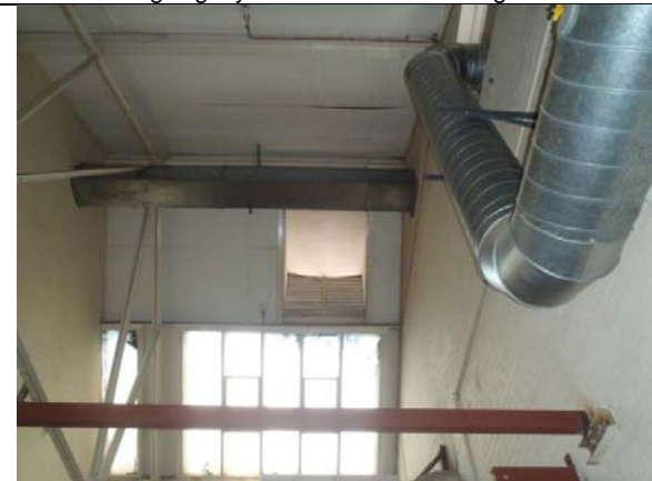
P17. The boarded roof, skylights and vent in the boiler room of Building 4.
