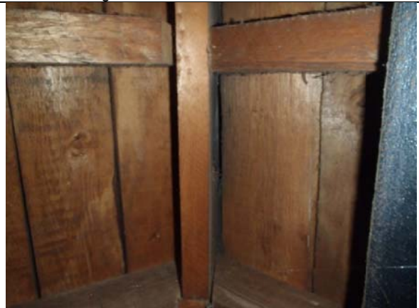
P12. The gap between the ridge and sarking boards in Building 3.
