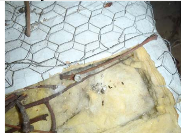
P5. Mouse droppings on the fibre glass at the south eastern end of the roof in Building 2.
