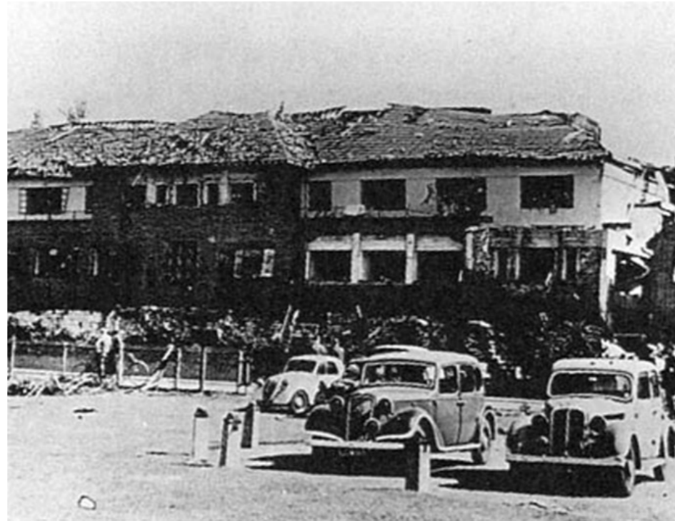
Figure 10: 1944 photograph showing the Administration Block of Teddington Studios after the explosion of 5 June. While the rear of the block was destroyed, the main facade stayed mainly intact, and was largely retained in its reconstruction.
