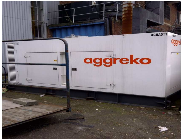
Image 12: Generator in the car parking area in the south-west of the site
