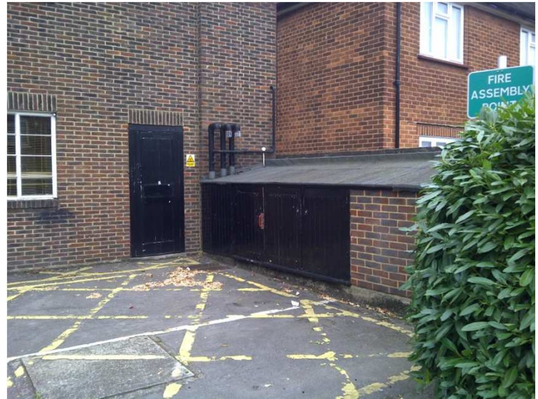
Image 2: Car park and side of the main building showing vent pipes
