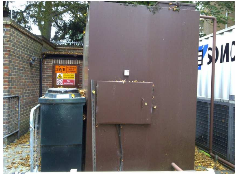
Image 4: Fuel tank located on the north-east
