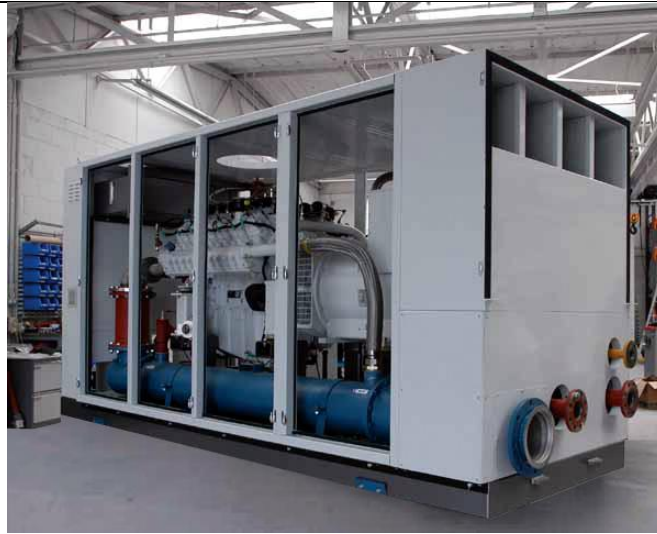
Energy Centre - Combined Heat and Power Unit
