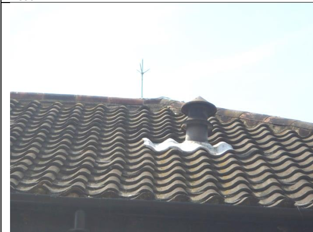
P9. Occasional gaps under roof tiles above sections of lead flashing on the north eastern side of the roof of Building 3.
