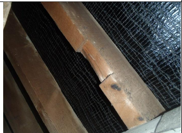
P6. The exposed bitumen and hessian felt at the south eastern end of the void.
