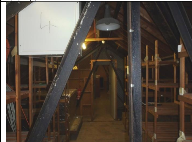
P11. The roof void in Building 3 showing the small enclosed room at the north western end of the void.
