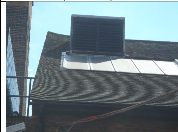
P15. The tiled roof of Building 4 viewed from the north west showing slightly raised tiles on the verge.
