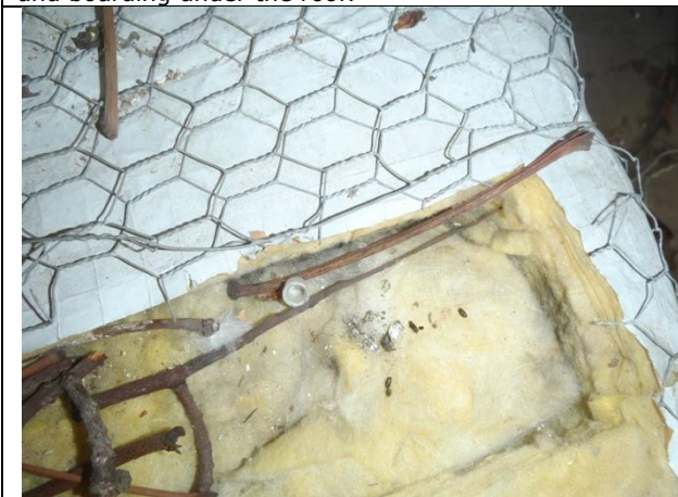
P5. Mouse droppings on the fibre glass at the south eastern end of the roof in Building 2.
