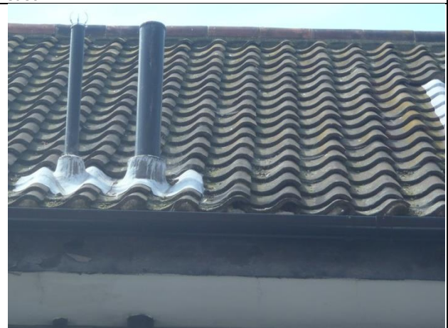
P10. Further occasional gaps under roof tiles above sections of lead flashing on the north eastern side of the roof of Building 3.
