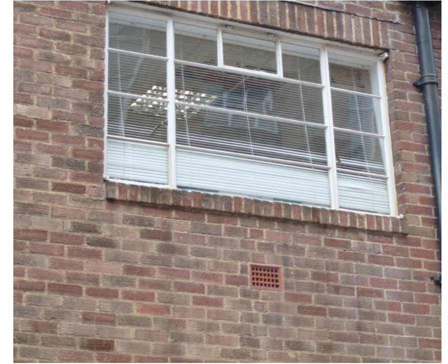
Figure 12: Photograph of the brickwork of the Administration Block's rear façade, of between 1944 and 1948, following the building's reconstruction.
