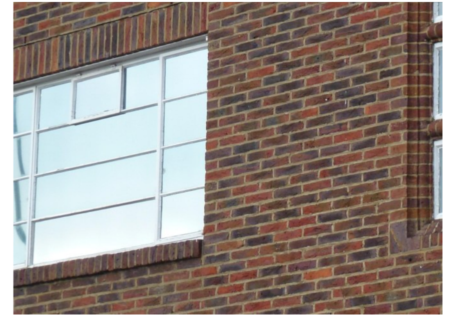
Figure 13: View of the front of the building, showing the very different original brickwork of the 1930s.
