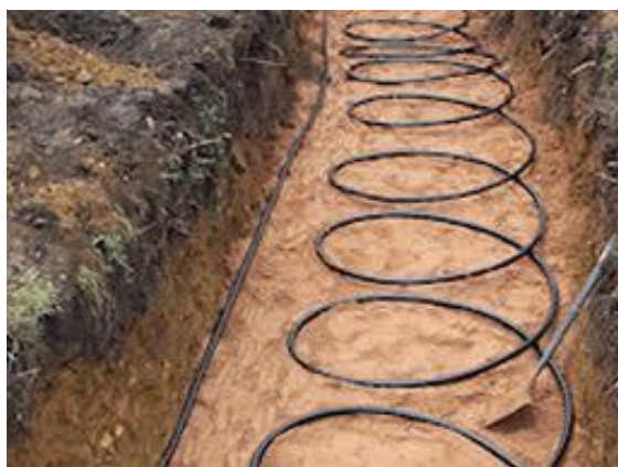
Image 2 – Ground sourced heat pump
