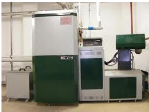
Image 6 – Combined Heat & Power Boiler
