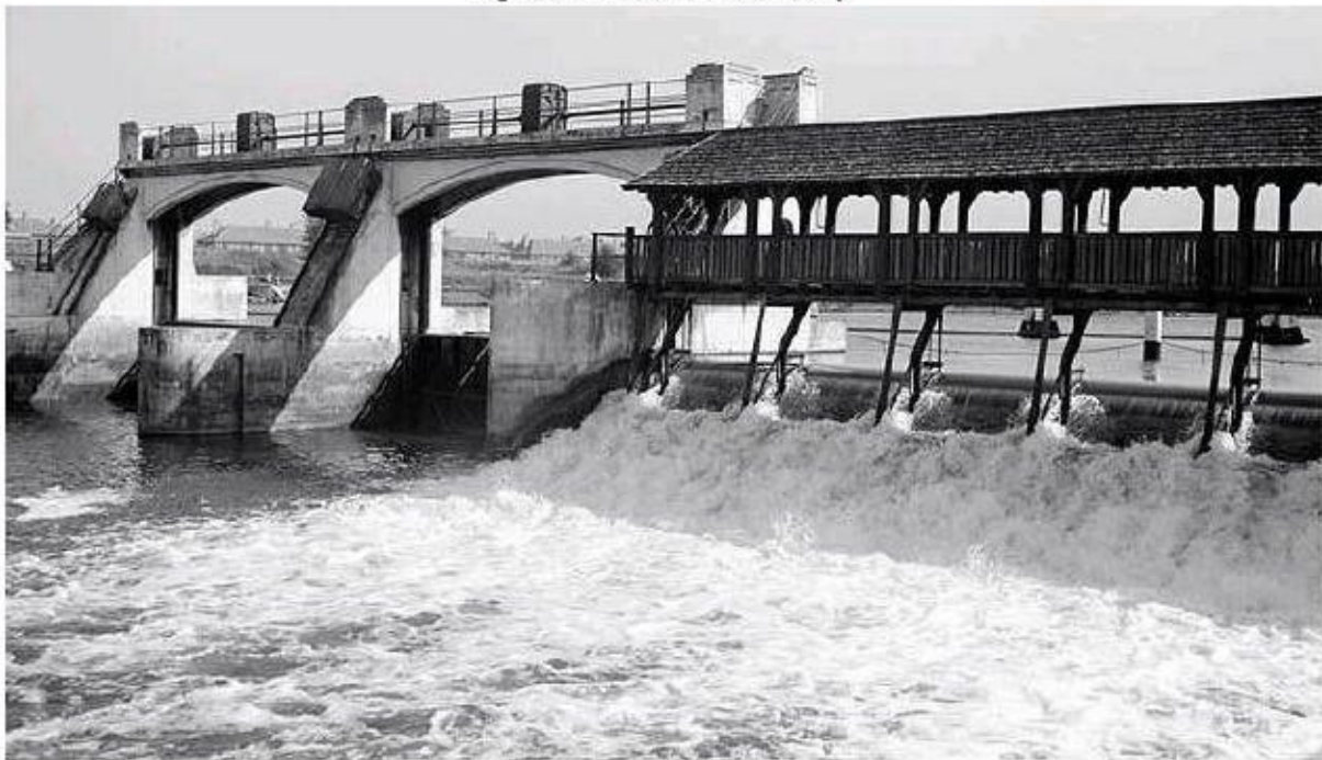
Fig 2. View of the relevant section of the weir, showing the former roofed walkway and overspill
