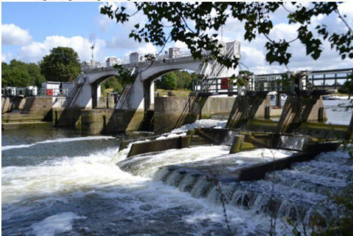
Fig. 4 Current view of the relevant section of the weir from the Teddington bank
