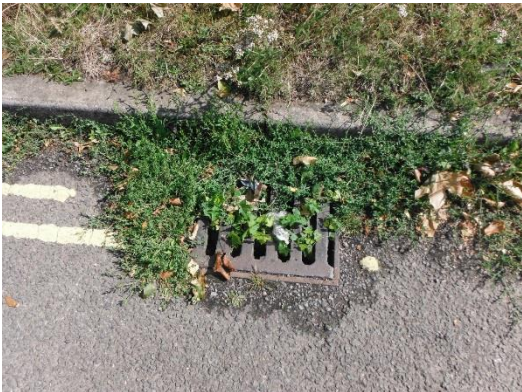
Figure 20 – Vegetated drain in Strathmore School car park
