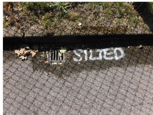
Figure 5 – Silted gully on Russell School entrance road
