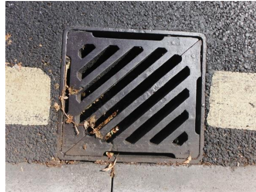
Figure 3 – Gully observed on Petersham Road
