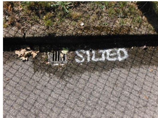
Figure 6 – Silted gully on Russell School entrance road
