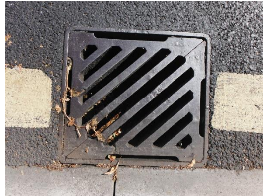
Figure 4 – Gully observed on Petersham Road
