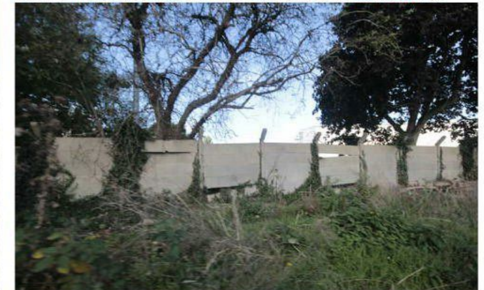
8. VIEW OF THE BOUNDARY TO THE WEST OF THE COUNCIL DEPOT, FACING THE DUKE OF NORTHUMBERLAND'S RIVER.
