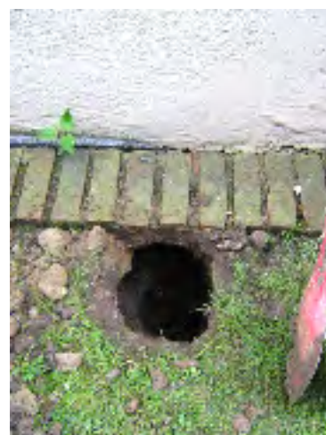
Photographic record of trial pit TP07
