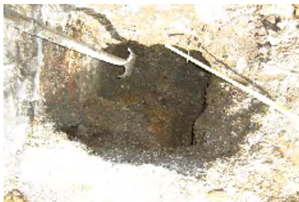
Photographic record of trial pit TP10
