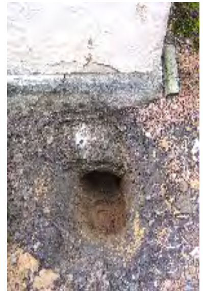
Photographic record of trial pit TP06
