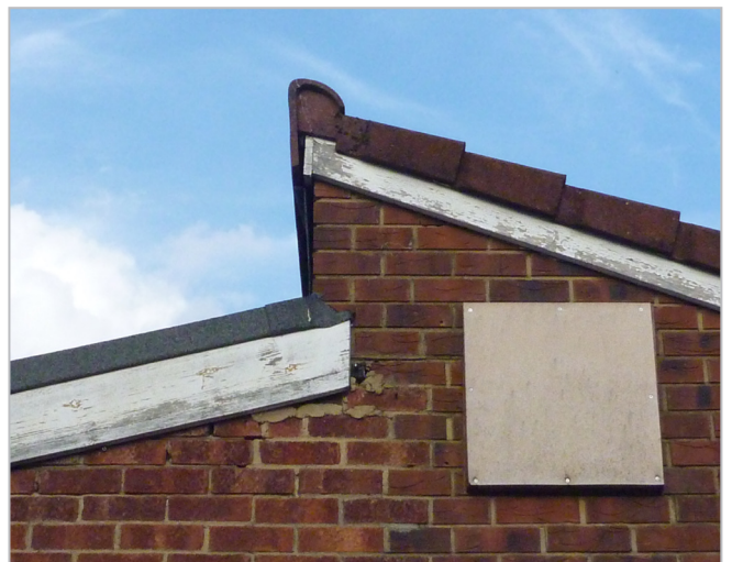
Photo 6 - gap behind fascia and tiles
