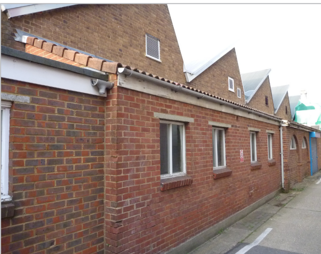
Photo 5 - holes in soffit
