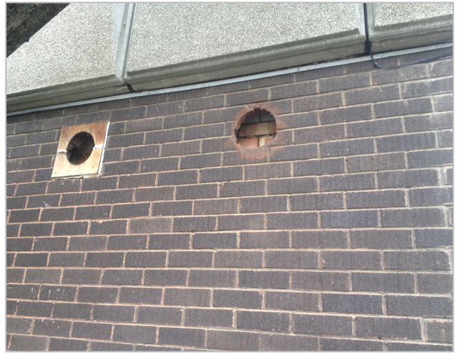
Photo 2 - holes in brickwork
