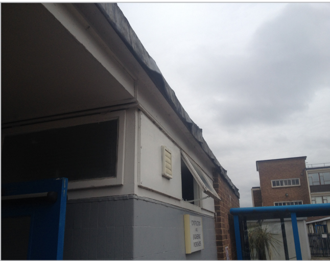
Photo 3 - lifted roof covering
