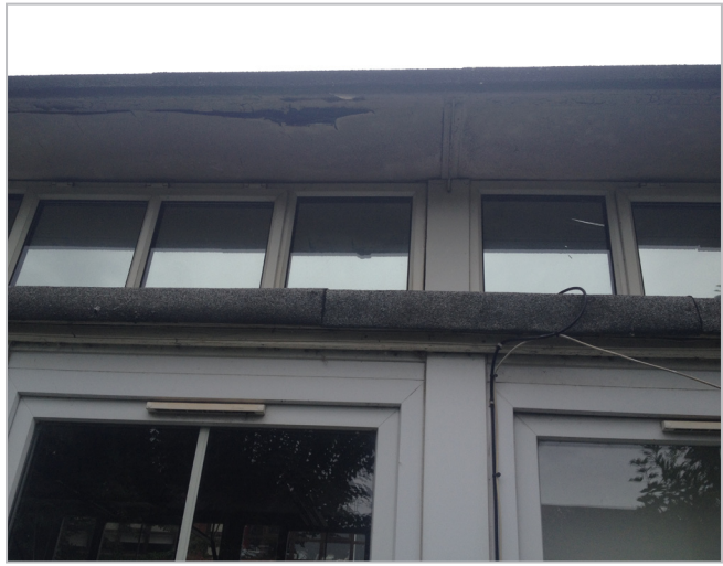
Photo 8 - Hole in soffit
