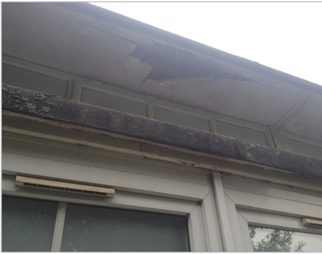
Photo 7 - Hole in soffit
