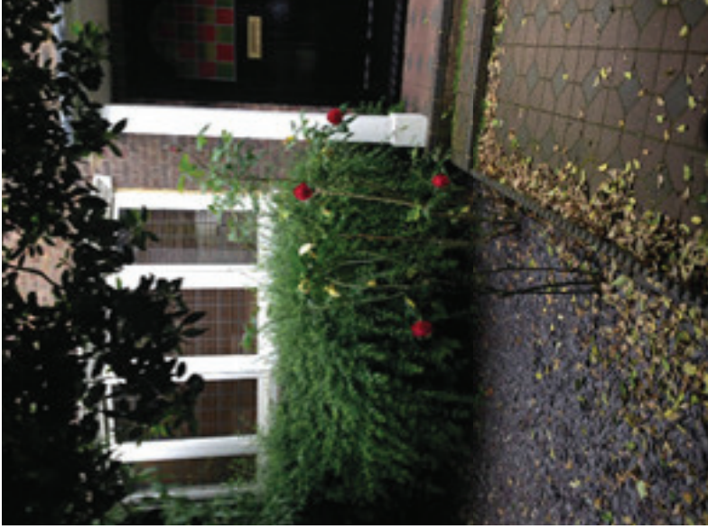
View of bay window & conservatory illustrating difference in level between Ground Floor & Ground Level
