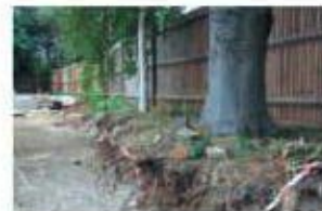
Potential loss of existing tree due to poor construction techniques.
