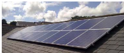
PV Panels mounted above tiled roof
