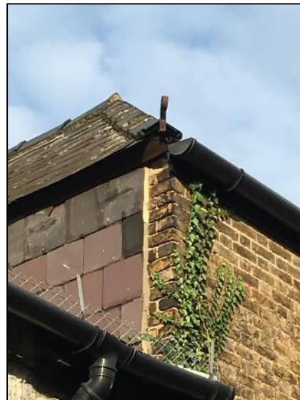
Photograph 8: Gap at eaves on western elevation of section that houses the organ
