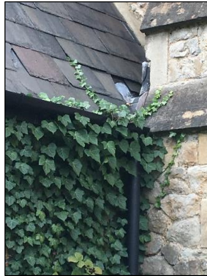
Photograph 6: Gap in roof tiles on eastern elevation of south porch entrance
