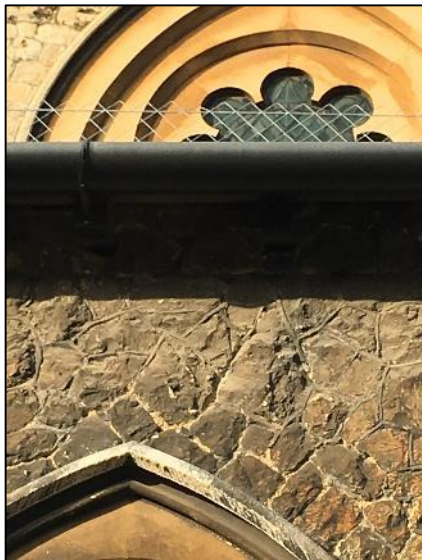
Photograph 7: Gap under exposed timbers on southern elevation
