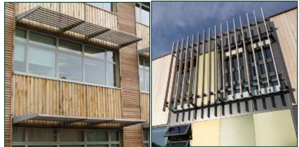
Figure 6. External solar shading 4
