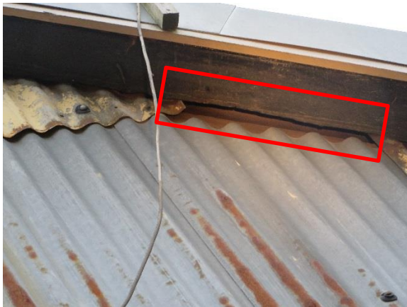
Photo 2- Gap underneath Soffit
