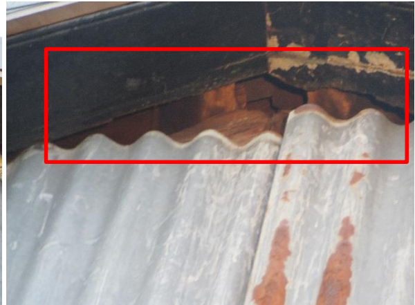
Photo 3- Gap underneath Western Gable
