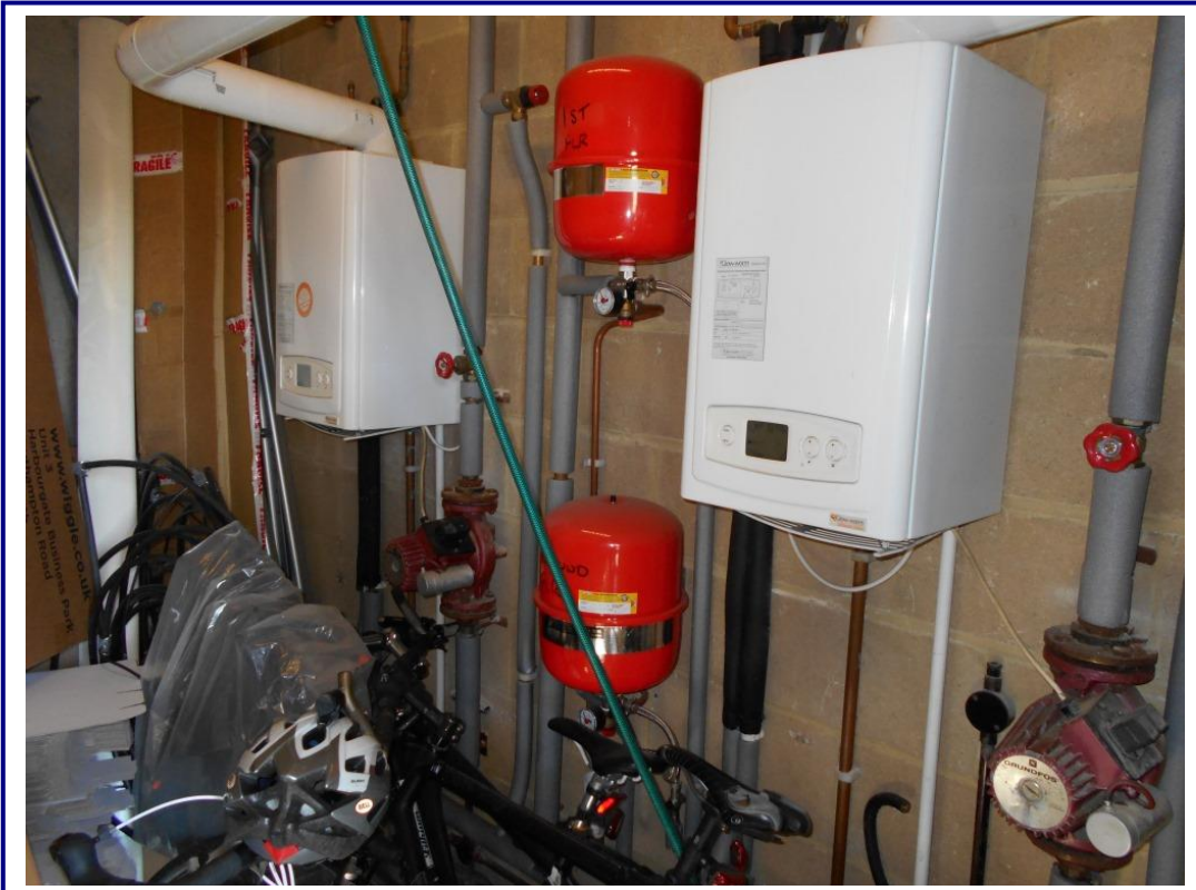
Photo 2: View of the natural gas boilers within a room off the undercroft car parking.
