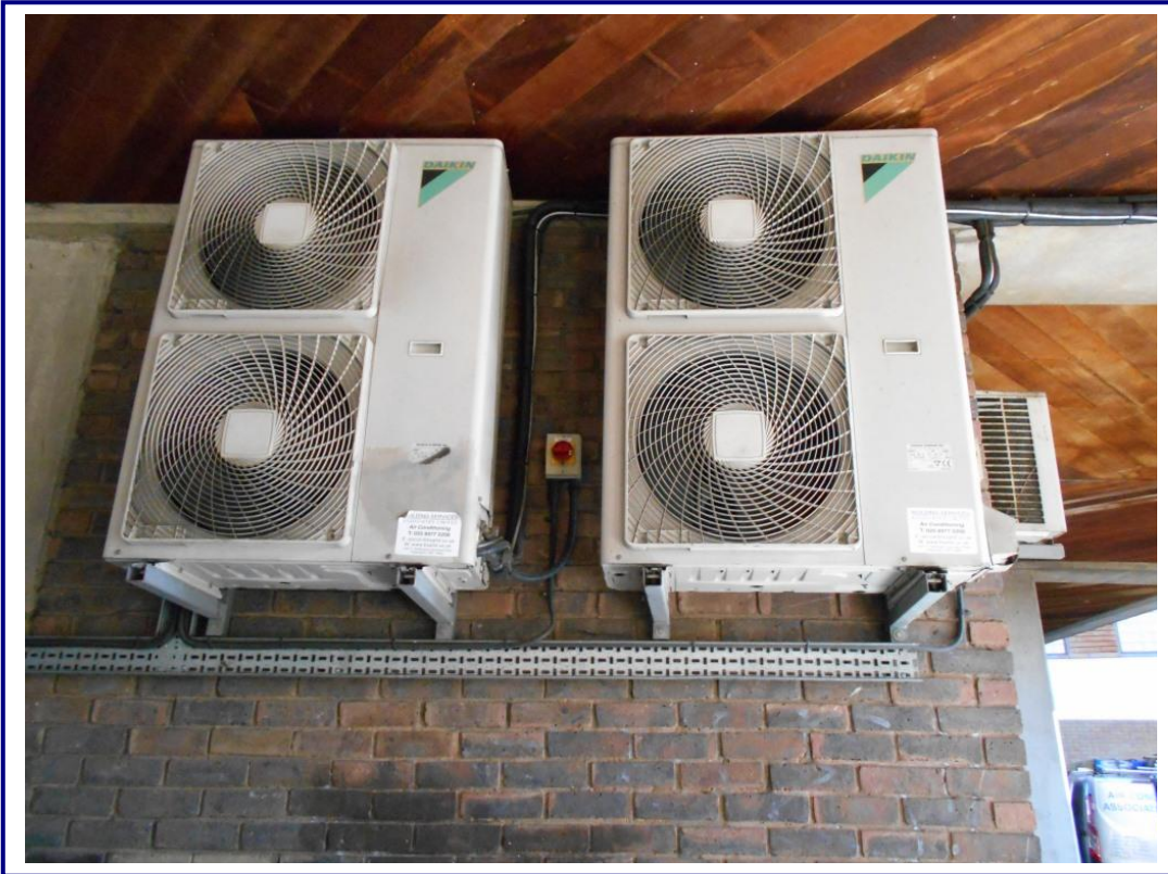
Photo 1: Air conditioning units within the undercroft car park.
