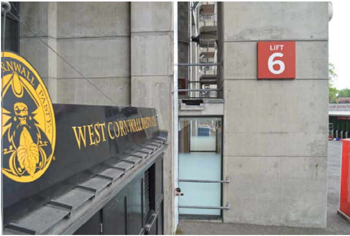
Photo 7 Concrete blockwork has no bat entry points
