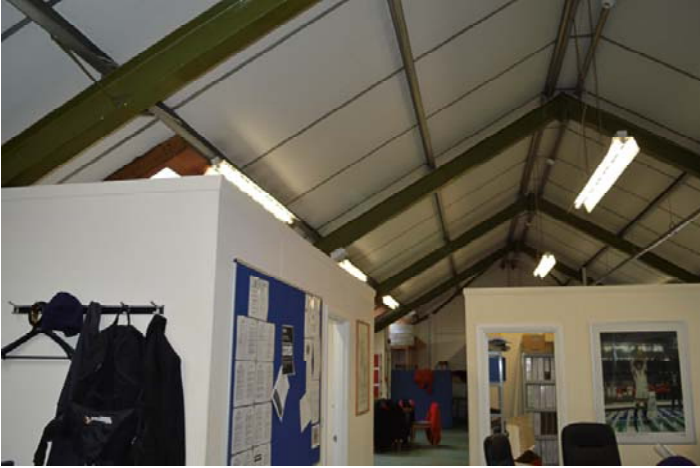
Photo 13 Internal view of maintenance shed showing boarding of roof with no loft spaces
