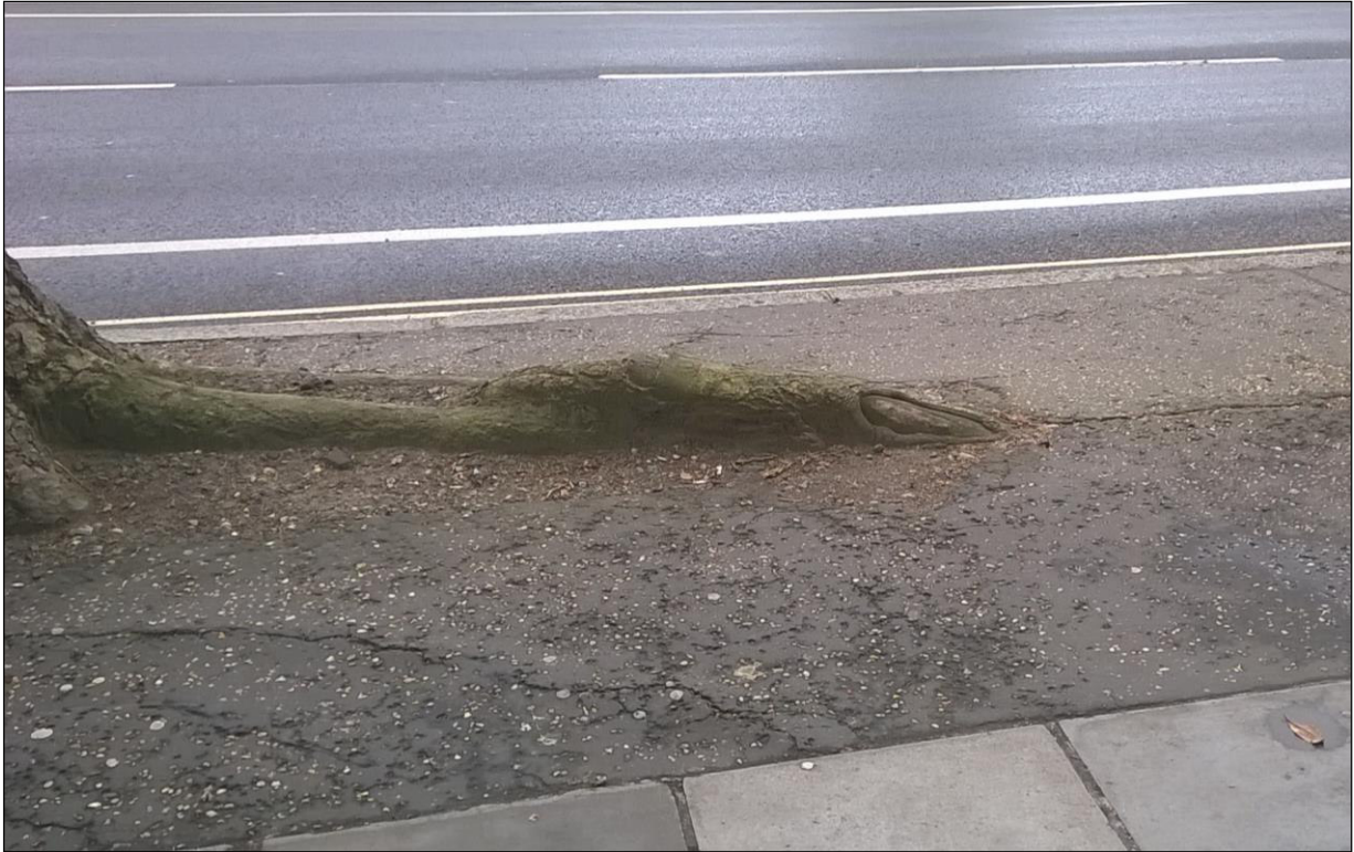
Image 2: Large surface root and obvious trip-hazard noted on T2 (Plane (London))
