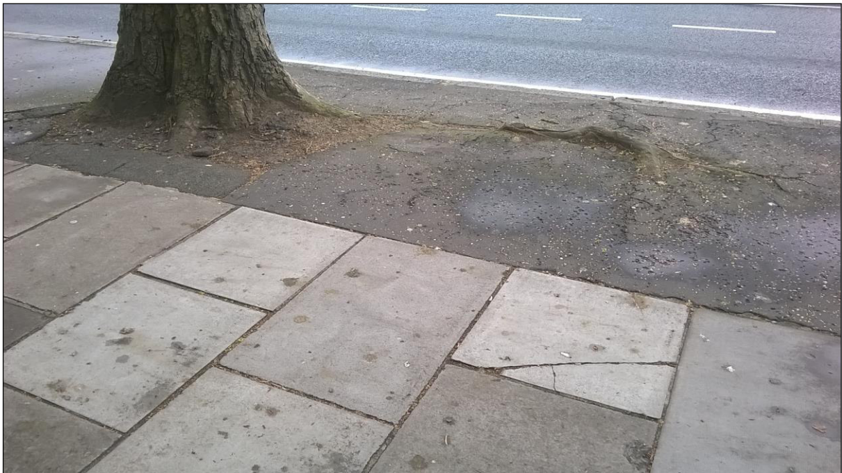
Image 3: Visible surface root and associated pavement damage from T3 - Plane (London)
