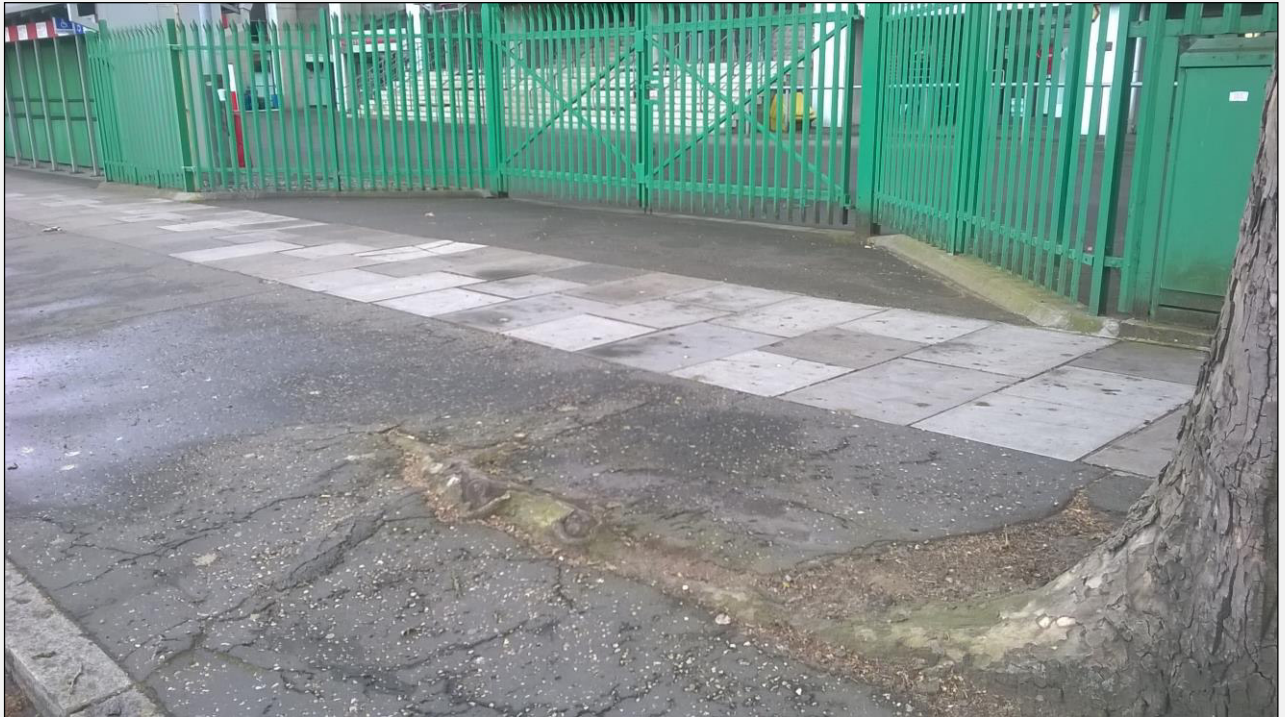
Location of T3 – Plane (London) opposite entrance gate; note visible surface roots, pavement damage and potential trip hazard.
