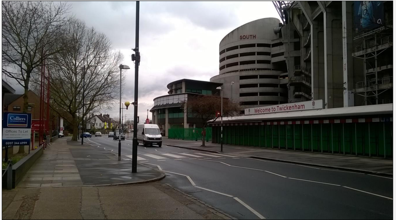
General Site Looking South towards Whitton Road with T6 on the left
