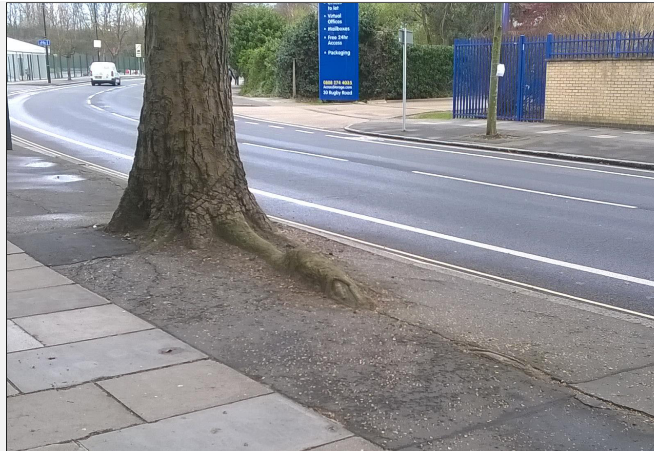
Large buttress roots and associated pavement damage observed near T2 – Plane (London)
