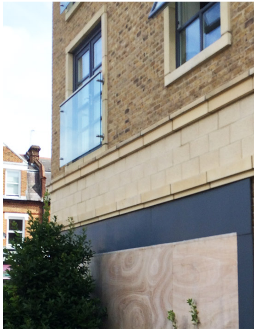
CRUDE DETAILING AND EMPTY SHOP UNITS
