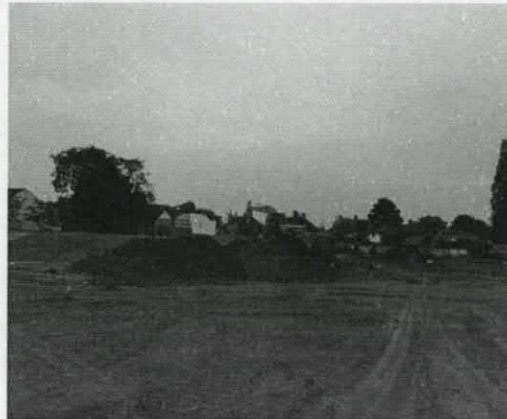
Contaminated stockpiles on bunded membrane
