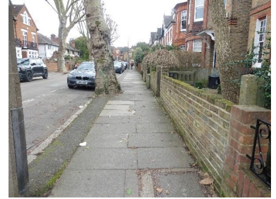
Link 20 – Radnor Road (Eastern footway)
