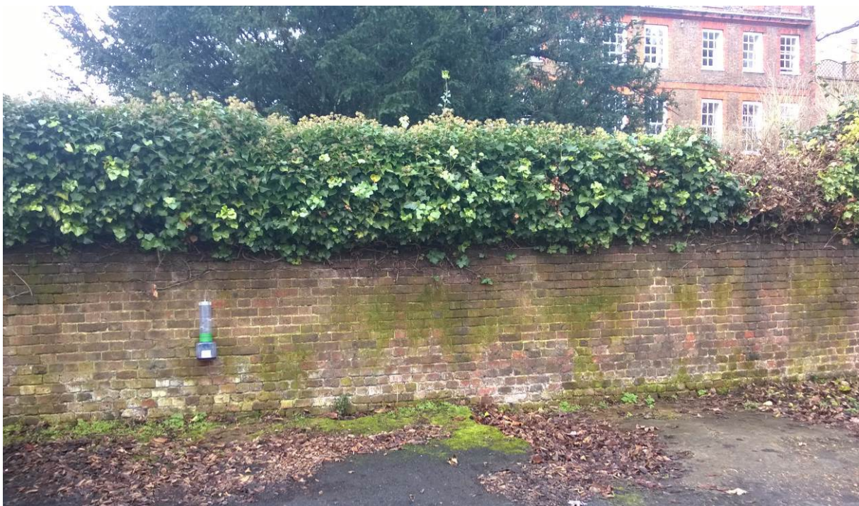
Photograph 10 – Extensive ivy growth to top of wall.
