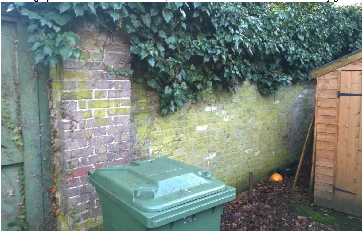
Photograph 24 – South end cross wall, height of wall increases, extensive ivy growth to top of wall.
