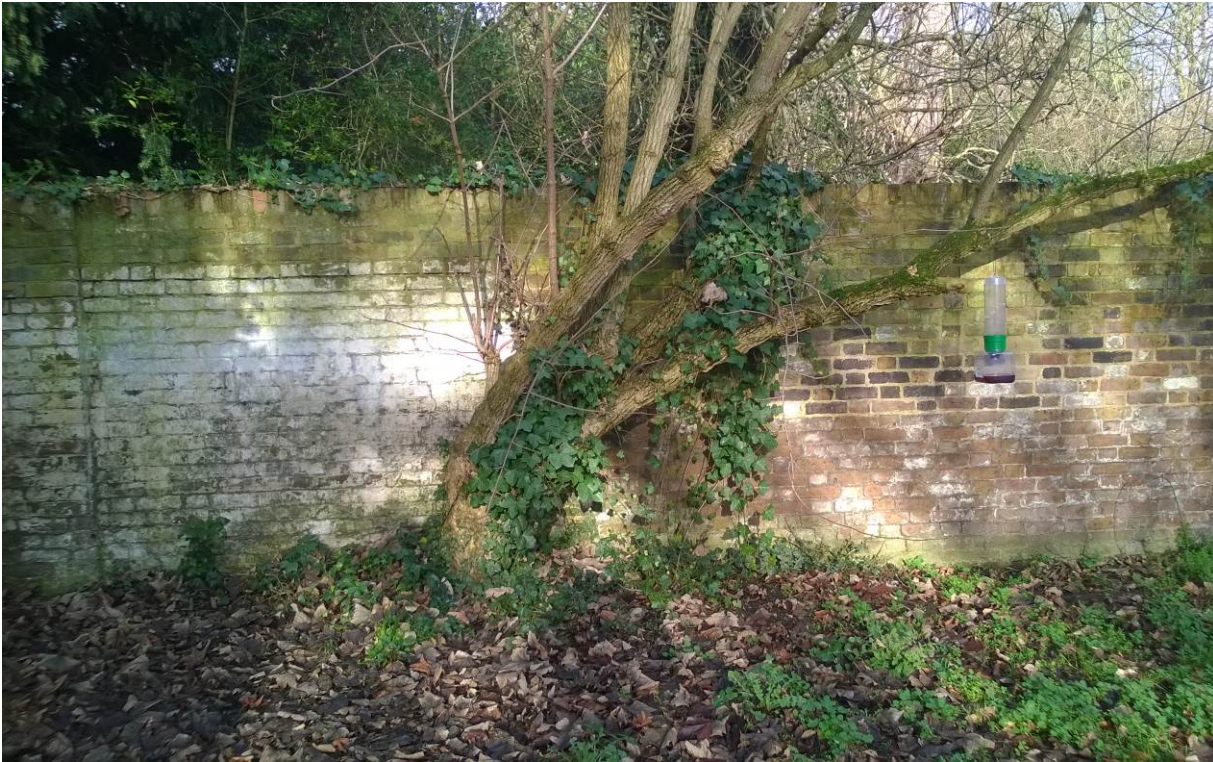
Photograph 17 – Elder tree in close proximity to north cross wall.
