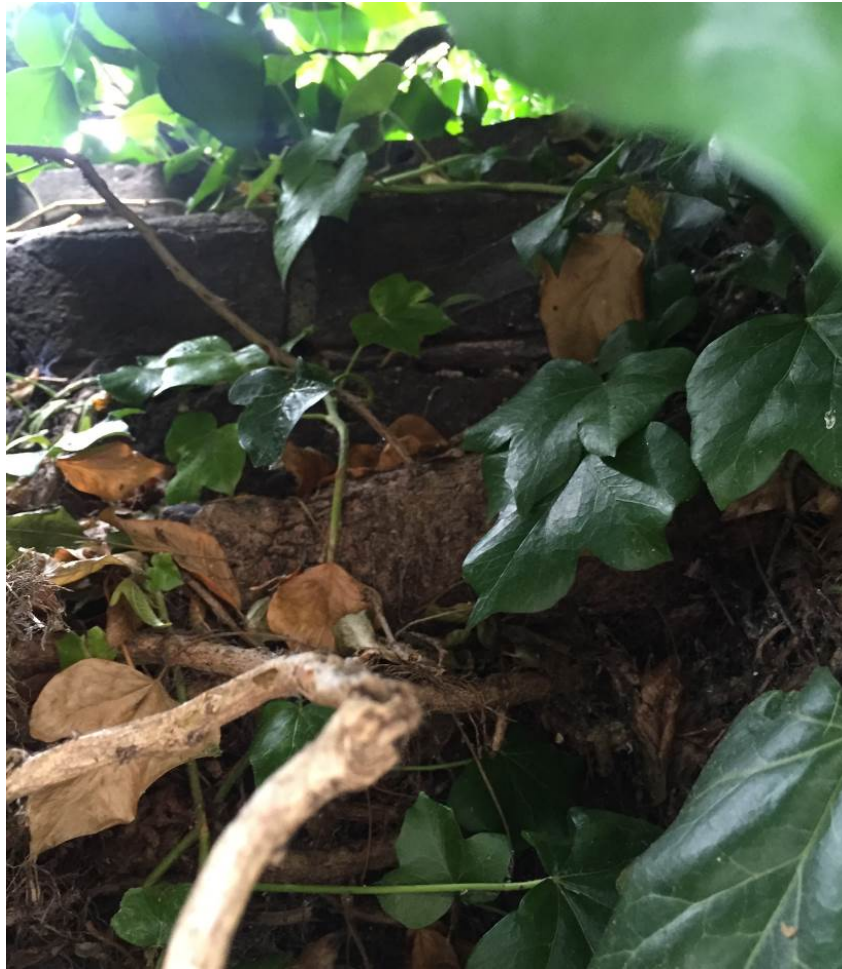
Photograph 9 – Vegetation growth and cementitious mortar has destabilised the top of the wall.
