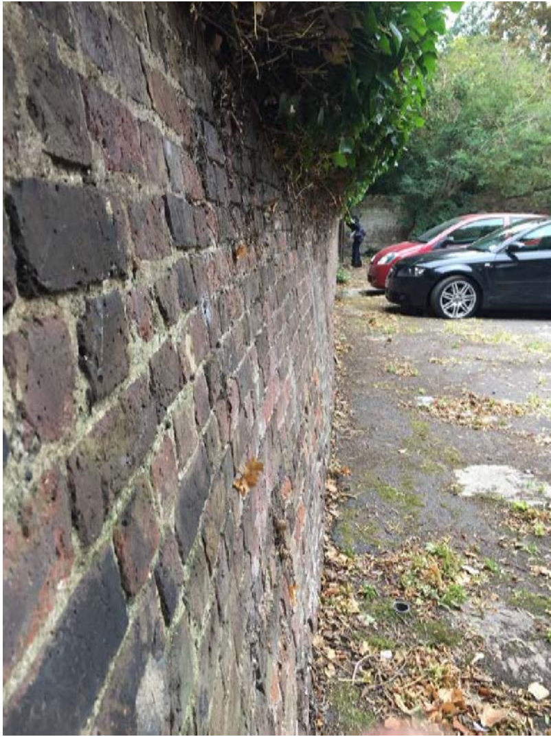
Photograph 7 –The severe lean in wall as viewed from the south end of the wall.
