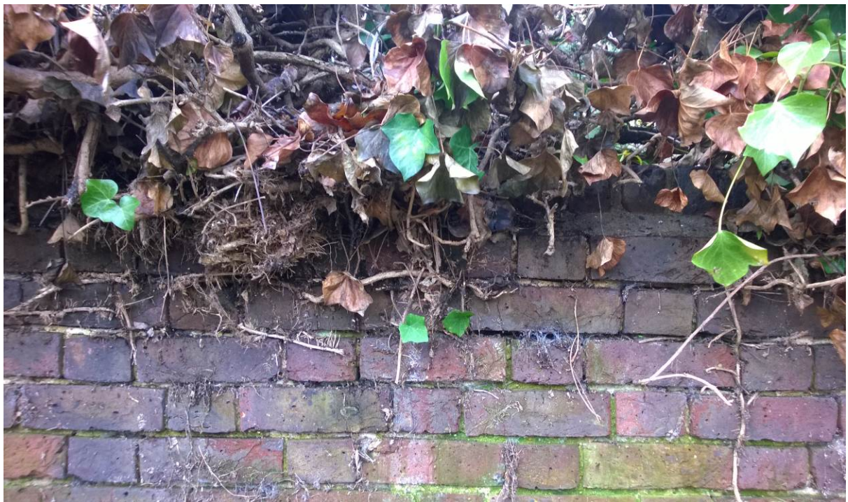
Photograph 14 – Root penetration into masonry at north end of wall.
