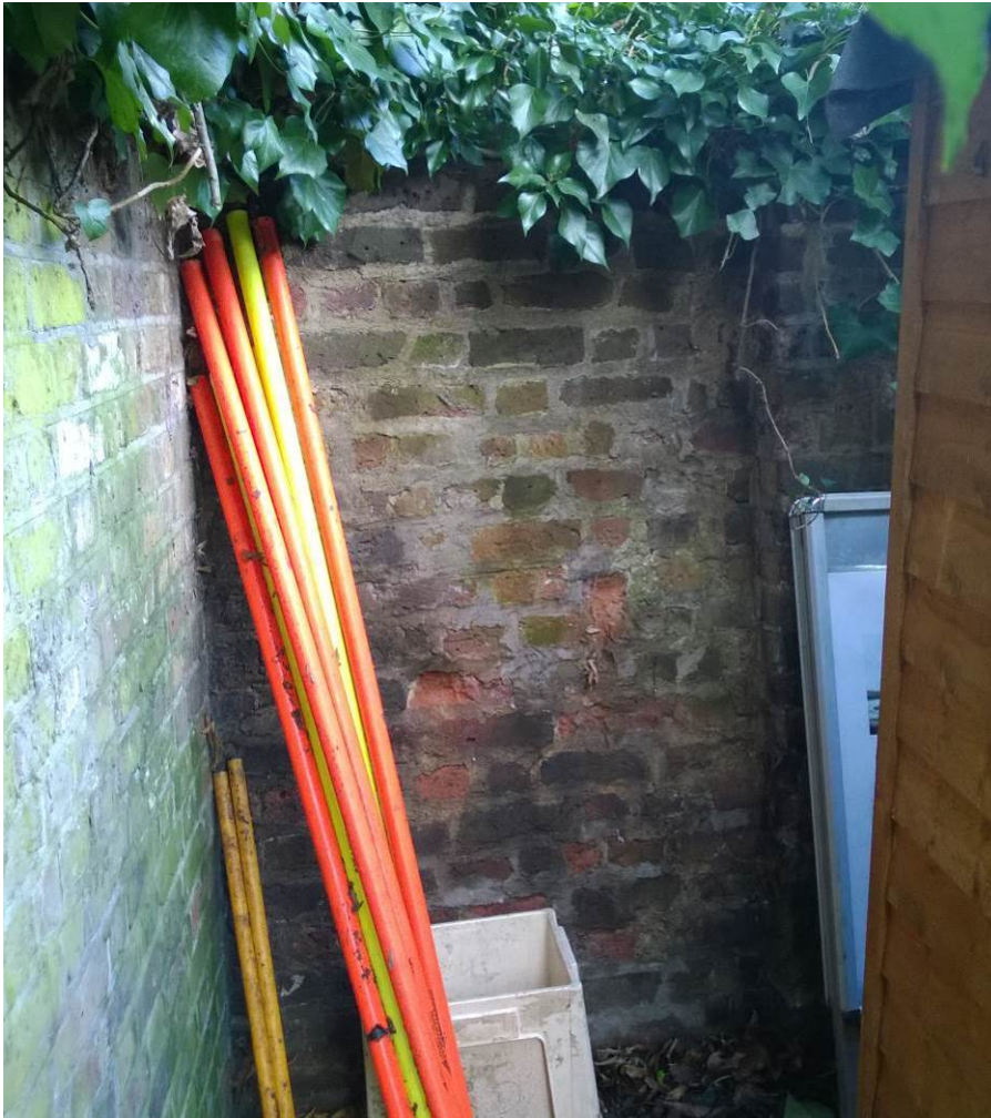
Photograph 23 – South end of main wall, minor erosion of bricks and extensive ivy growth.
