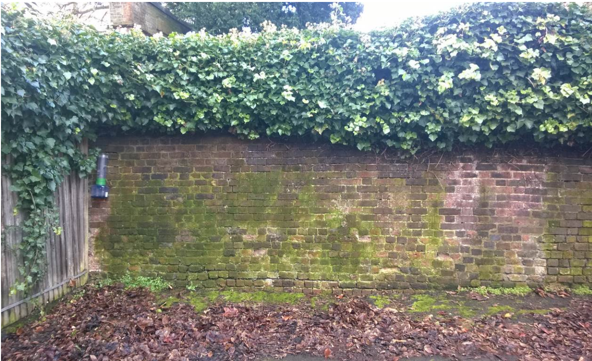
Photograph 4 – South end of wall, wall severely bowed in this area.
