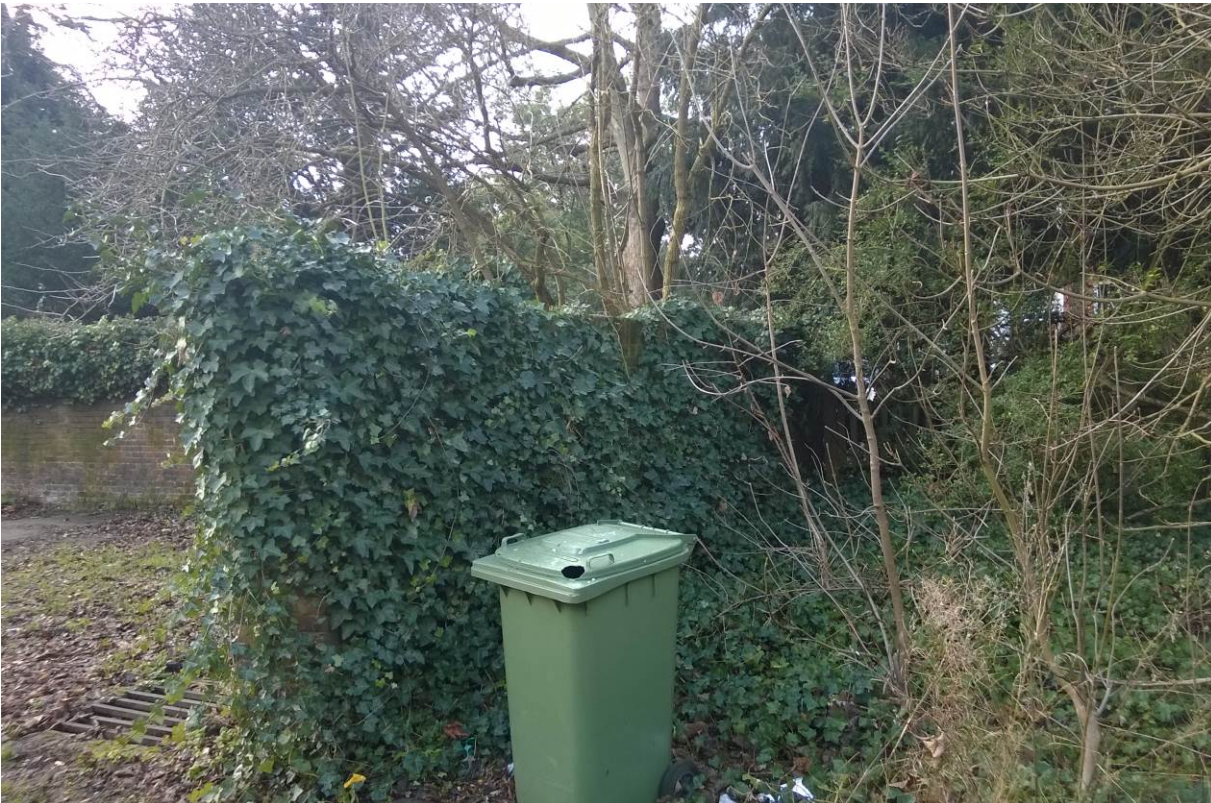
Photograph 20 – Ivy growth to north elevation of north end cross wall.
