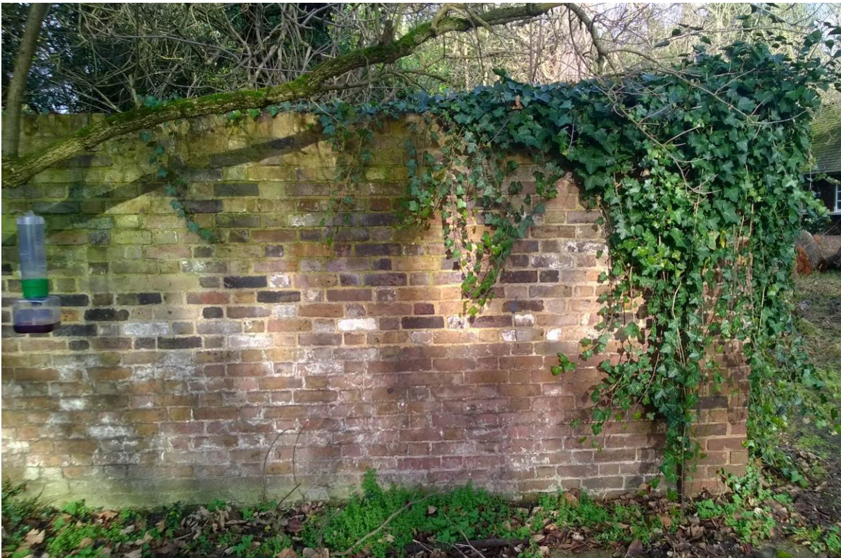
Photograph 18 – Ivy growth to north cross wall.
