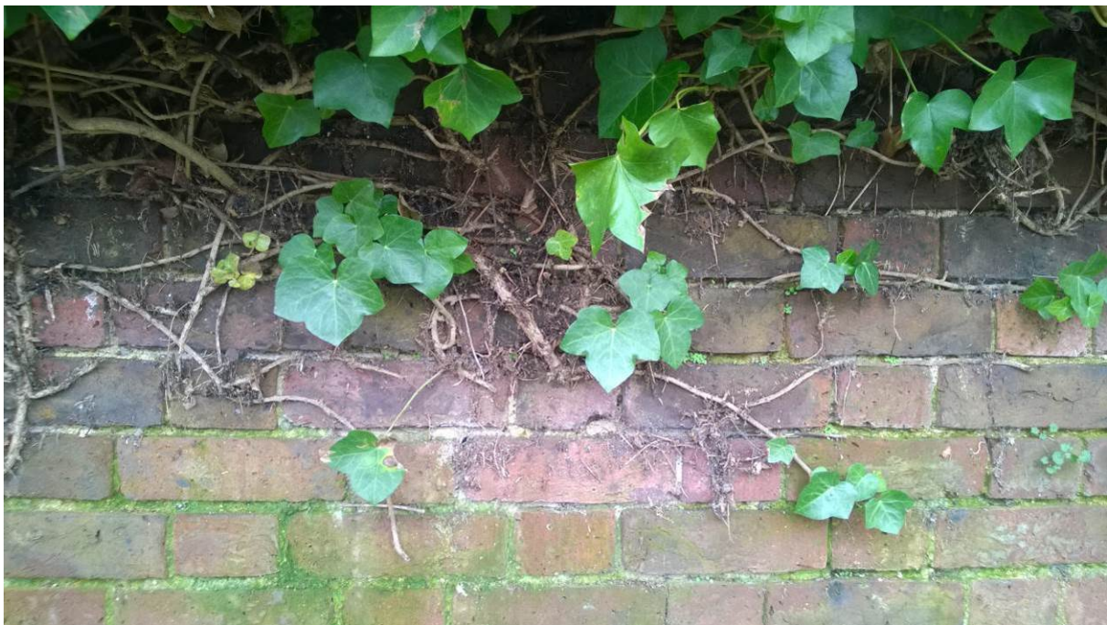
Photograph 12 - Root penetration into masonry to top of wall.
