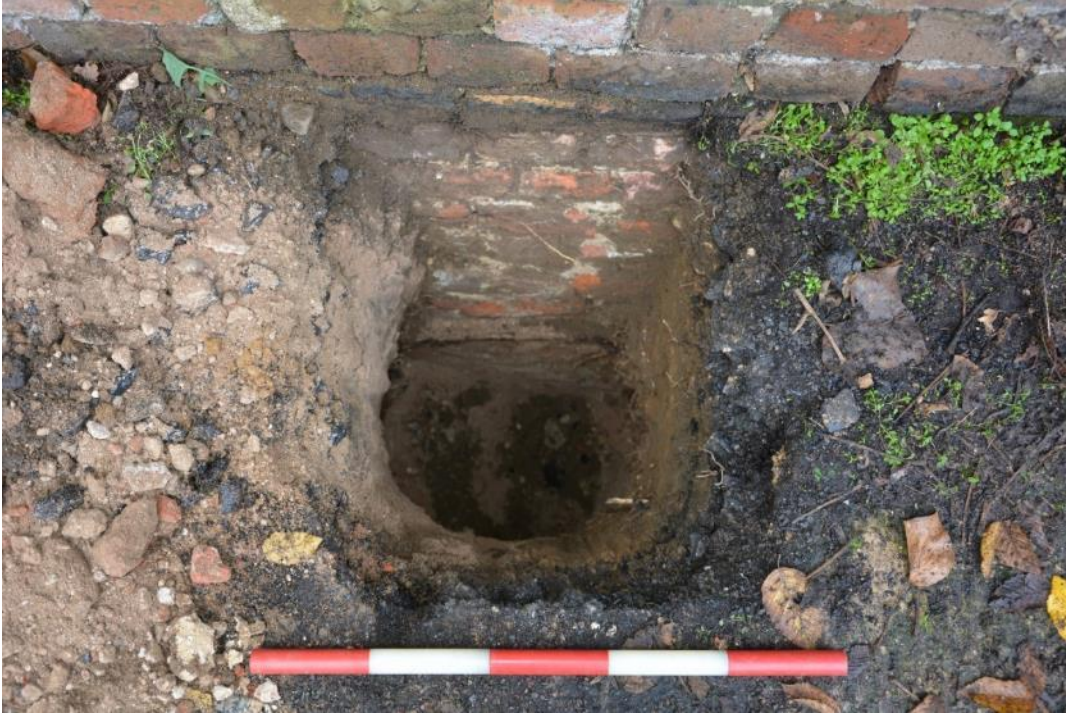
Figure 14: TP3 - exposed footings, significantly deeper than those exposed in TP1. Facing W. Scale 0.5m.
