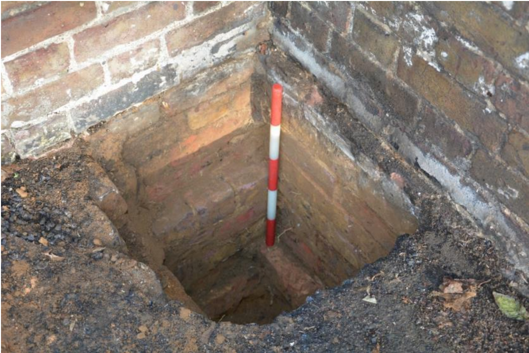
Figure 13: TP2 - exposed foundations of the modern, and coach house walls. Facing NE. Scale 0.5m.
