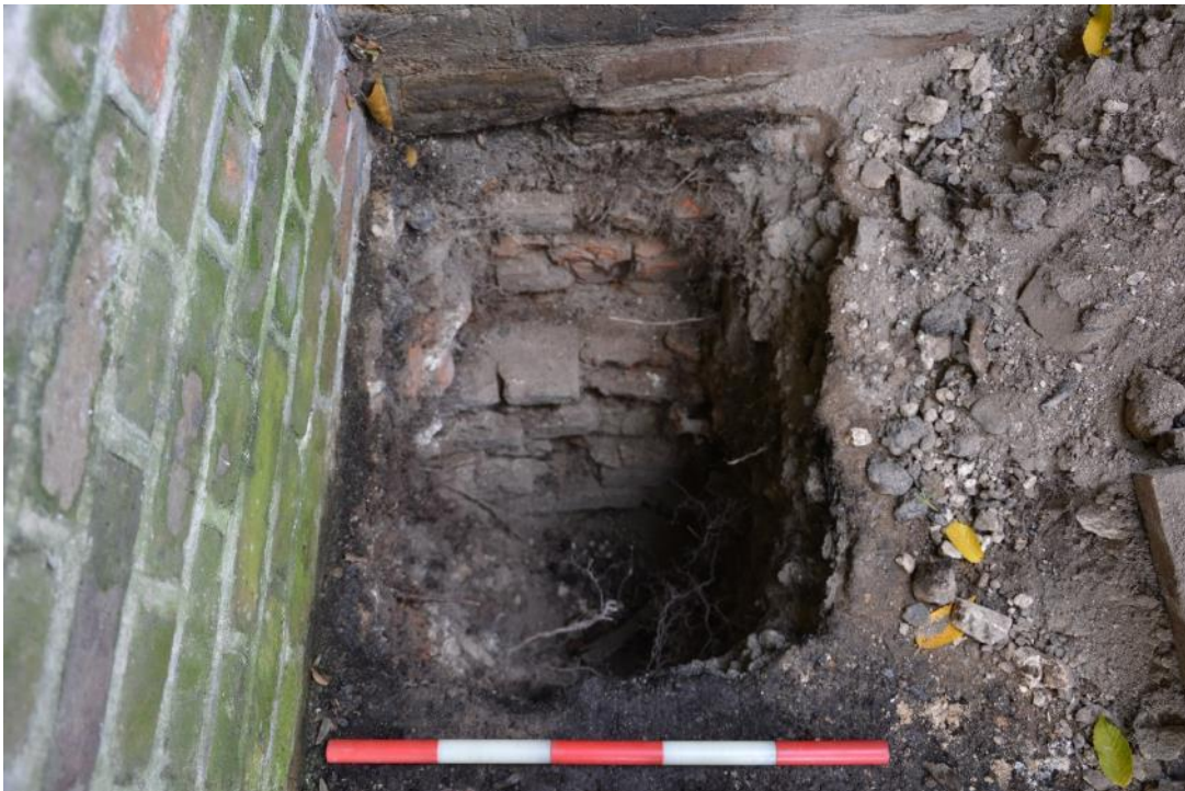
Figure 18: TP5 - extremely loose and fragmented foundations of the party wall. Facing W. Scale 0.5m.
