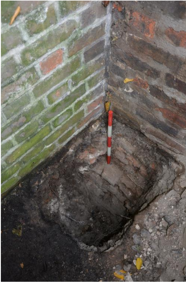
Figure 19: TP5 - crumbling foundations and rubble abundant backfill below macadam surface. Facing SSW. Scale 0.5m.
