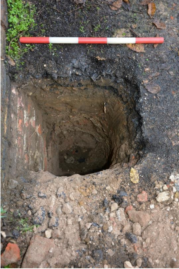
Figure 15: Stratigraphy of the SSE facing section, showing the macadam (3) above compacted silty clay (7), loose demolition material (8) and natural at the base (9). Facing approximately NW. Scale 0.5m.
