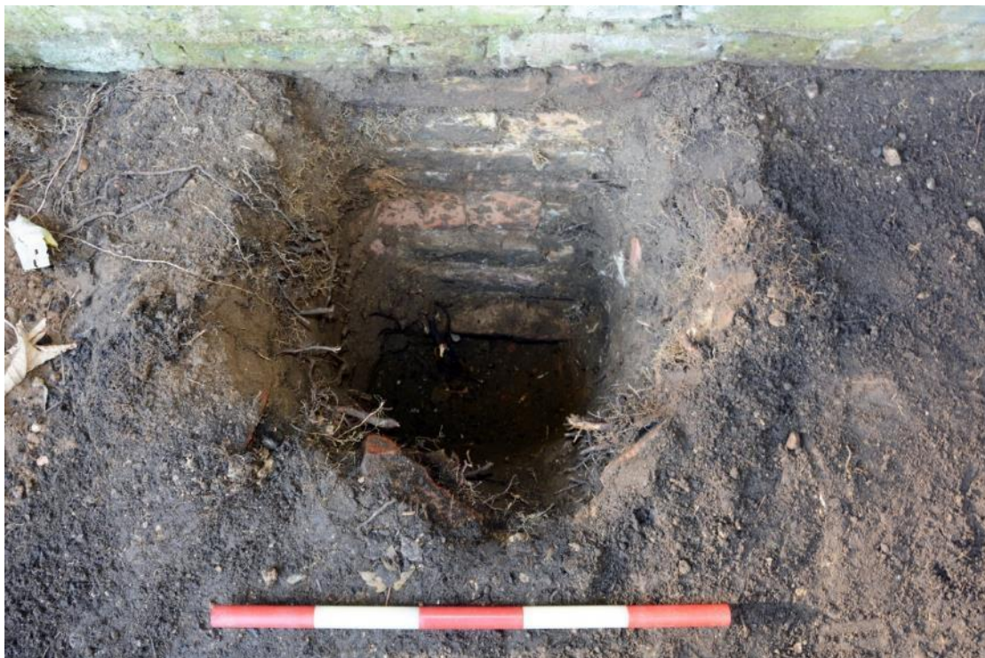
Figure 11: TP1 - exposed foundations of existing N-S party wall. Facing W. Scale 0.5m.
