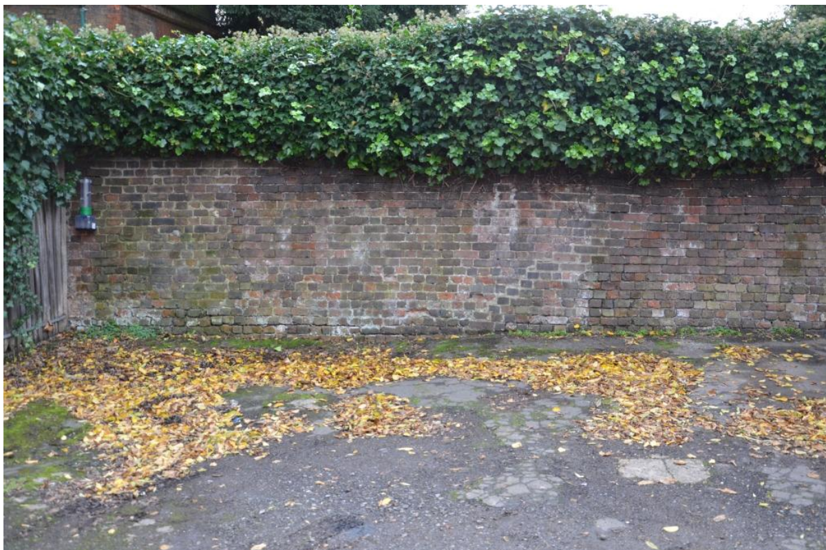
Plate 3 Southern end of the long western yard wall showing repaired crack and slumping to the north. Viewed from the east
