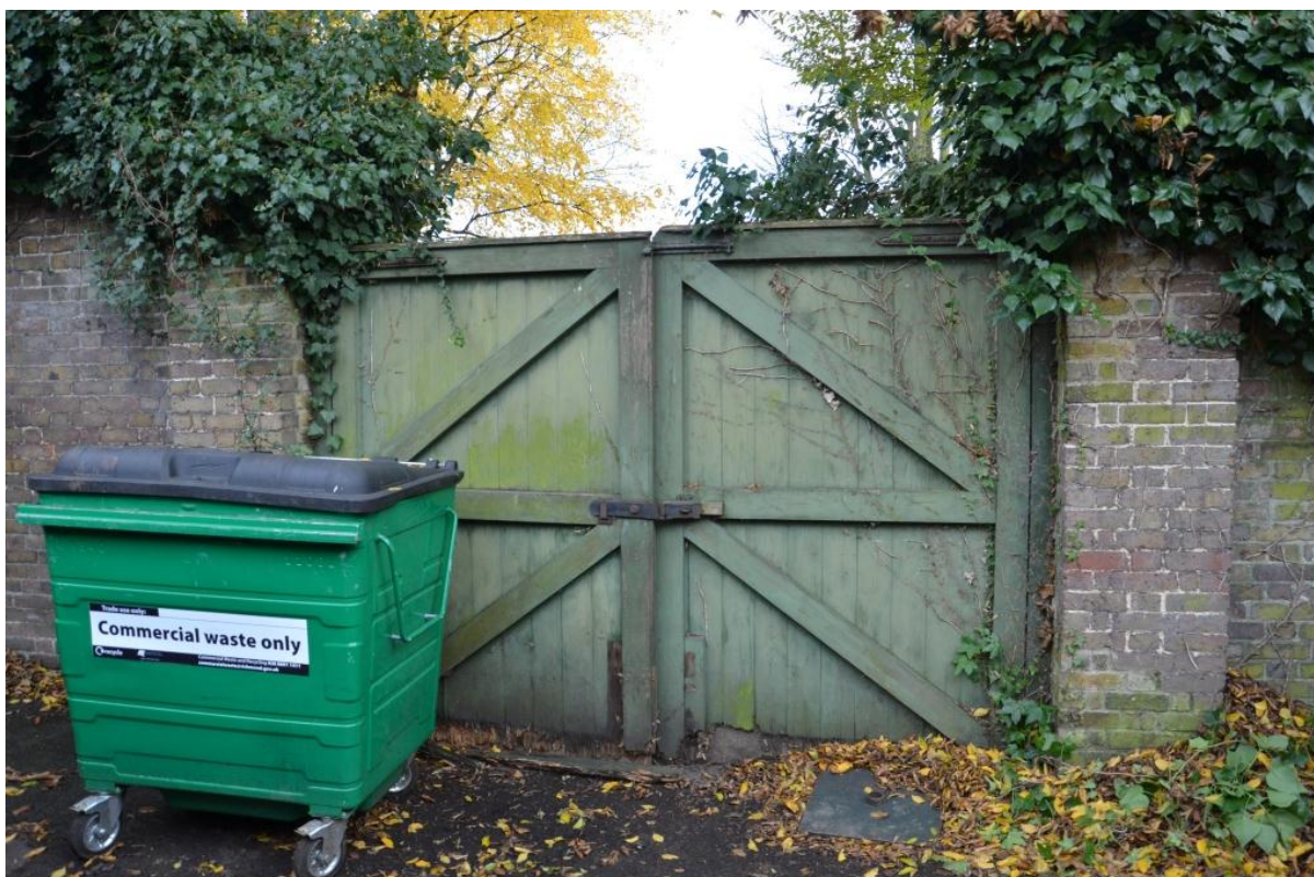
Plate 8 Gate piers framed by the southern return of the yard wall; internal view from the north.
