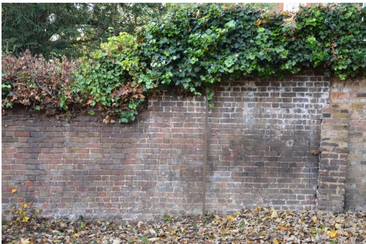
Plate 4 Northern end of the long western wall showing rise and buttress marking newer section to right.
