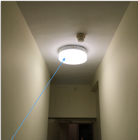
Fittings require no extra cabling and we are proposing replacing in same locations, using more decorative fittings to English Heritage spec
