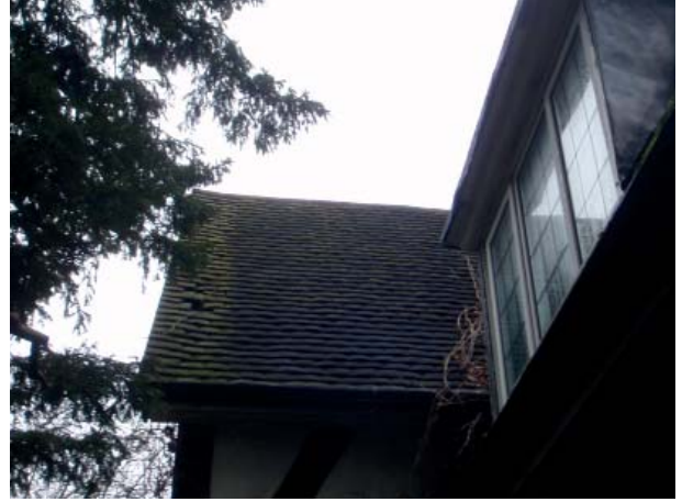
Plate 2. Section of roof with slipped/missing clay tiles.
