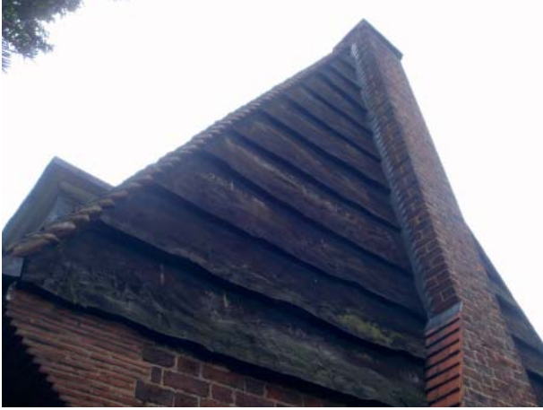
Plate 1. Weatherboarding with gaps on south-east gable end.
