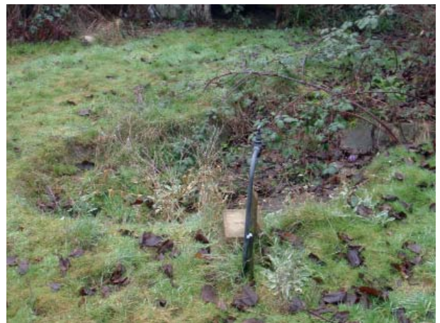
Plate 6. Dry pond lined with concrete slabs and encroaching vegetation.
