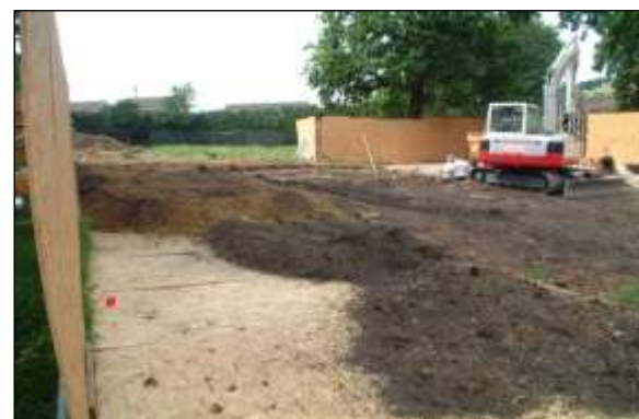
Ground protection image 2: Spreading soil excavated from footings is an effective way of buffering the plywood surface from the wear of light vehicles.
