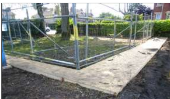
Ground protection image 3: Plywood fixed to a wood frame is another effective method of protecting soil from pedestrian compaction.
