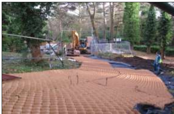
New surfacing image 2: The three-dimensional cells are opened up, spread across the area to be surfaced and pinned in place ready for the stone filling.
