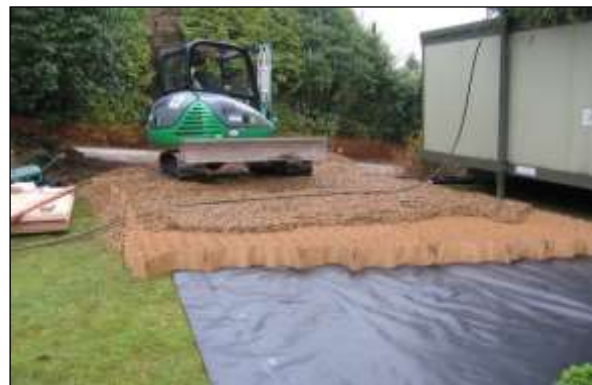
New surfacing image 3: The stone-filled cells spread the load of traffic and the geotextile membrane on the ground prevents migration of the stone into the soil profile.
