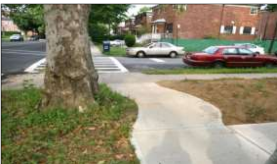
New surfacing image 7: In some situations, it may be appropriate to cast a free floating concrete surface directly onto the soil surface provided provision is made to prevent soil contamination while the concrete is being poured, i.e. an impermeable membrane separating the concrete from the soil.
