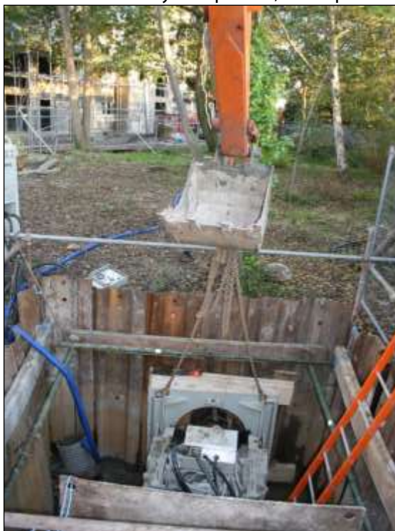
Services image 1: If possible, thrust boring is the preferred option for installing service routes through the RPAs of important trees, but there has to be space at the start and finish to dig substantial working pits.
