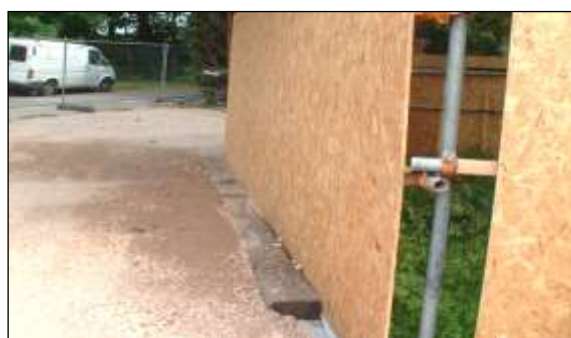
New surfacing image 5: Although this is only a temporary surface, railway sleepers pinned into the ground can be used to retain the edges of new surfacing.
