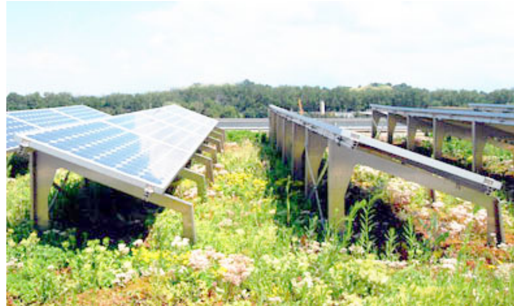
BROWN ROOF WITH PHOTOVOLTAIC SOLAR PANELS
