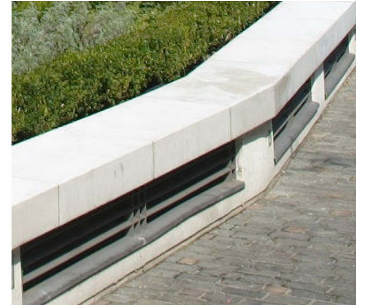
Integrated basement ventilation
